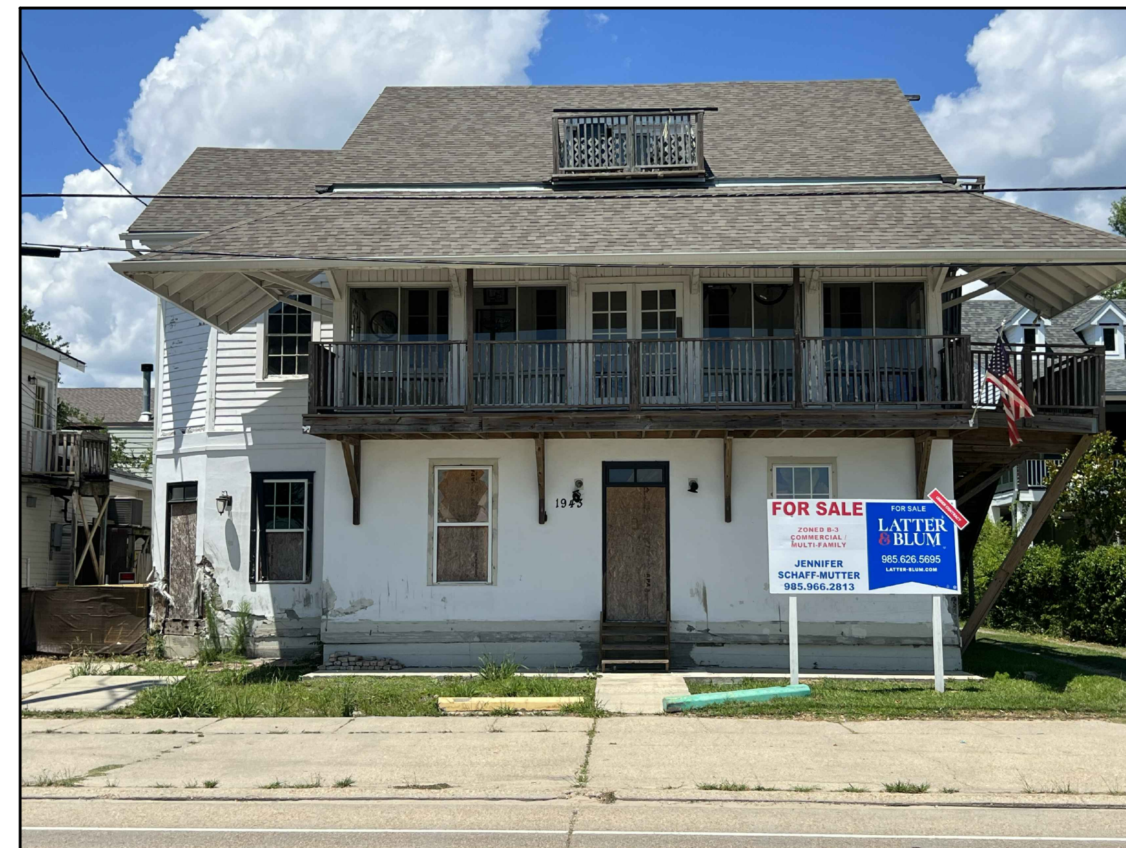
EXISTING BUILDING AFTER HURRICANE IDA
