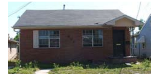
Porch does not meet minimum dimension requirements.
