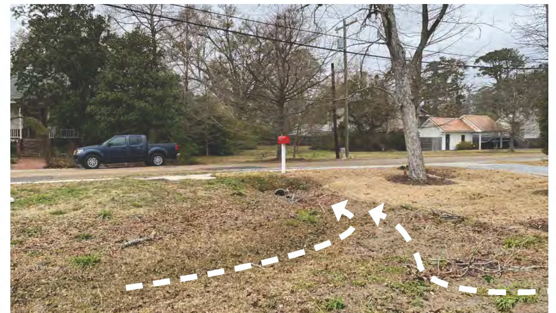
Ravine Aux Coquilles drainage pipe inflow & outflow on site
