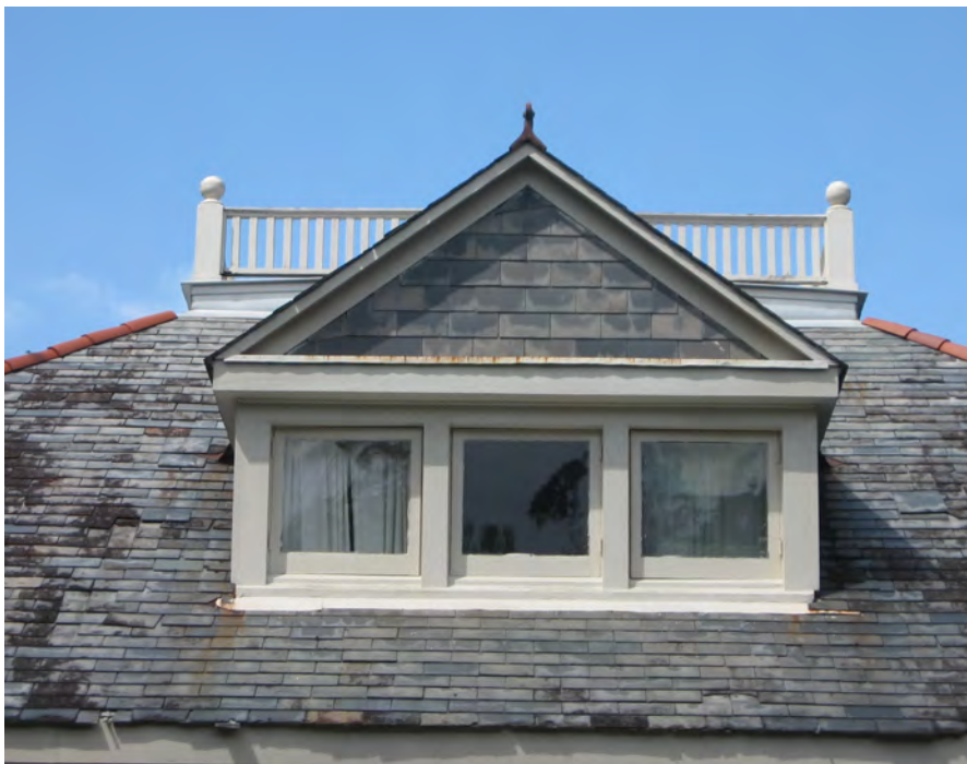
This original slate roof is a significant feature of the dwelling at 402 Lafitte Street and should be preserved.
