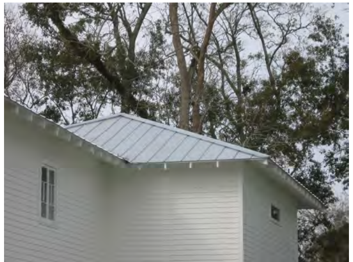
New standing seam metal roofs should be in traditional designs and spacing as at 132 Carroll Street.
