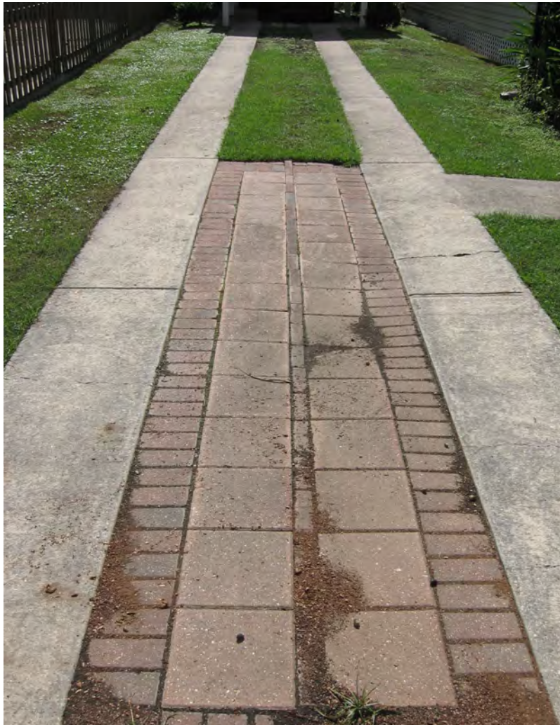
The concrete “ribbon” driveway at 1928 Monroe Street is a traditional design for driveways.
