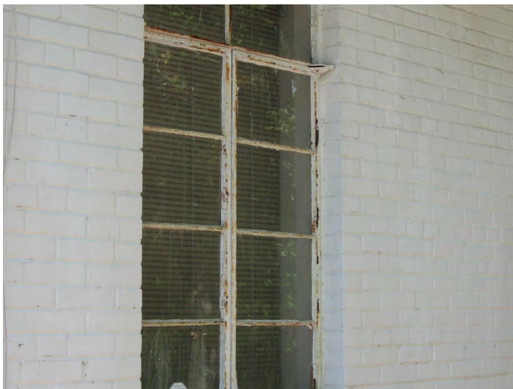
In addition to wood sash windows, steel casement design windows were widely used in the twentieth century (Jefferson Street).
