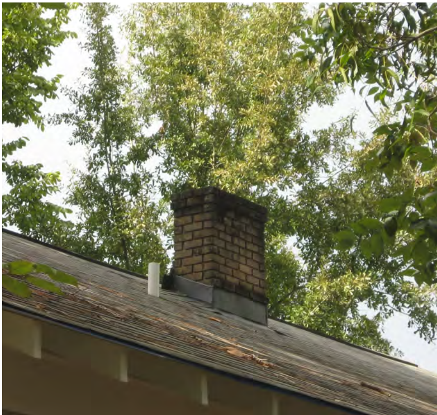
Most chimneys in Mandeville are built of brick and offer a textural contrast to frame dwellings (203 Girod Street).
