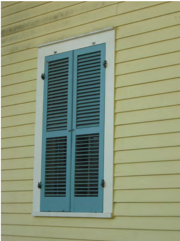
Window shutters should be sized to cover the exact dimensions of their windows, as at 317 Girod Street .
