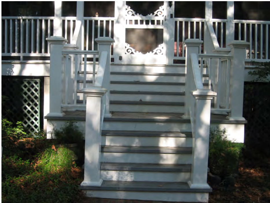
This rebuilt staircase is an appropriate example of wood construction with simple handrails and balusters (306 East Street).
