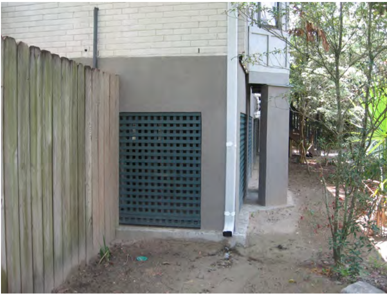
YES: Breakaway wood lattice panels appropriately placed within the piers of this elevated foundation.
