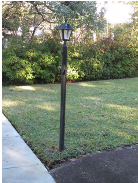
The installation of small footlights along walkways is appropriate for the historic district (right) as well as pole mounted light fixtures (above).
